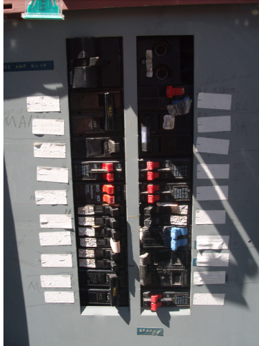
Figure 6: Existing 200A Service Panel
