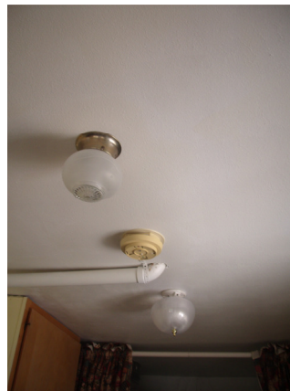
Figure 5: Typical Smoke Detector
