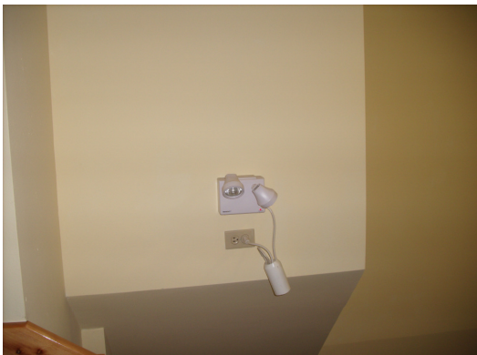
Figure 4: Emergency Light in Stairwell
