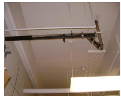
Acid waste resistant piping is in poor condition. There are visible leakages.
