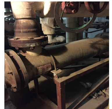
Chilled industrial water heat exchanger is in poor condition.
