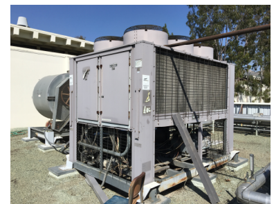
Abandoned air cooled chiller to be demolished previously serving chilled industrial water system.
