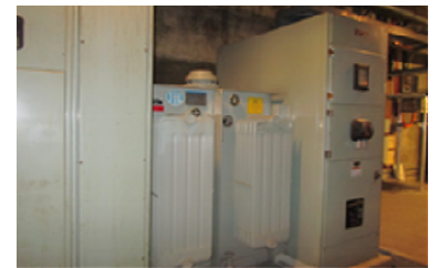
Existing Unit Substation #1 Transformer with PCB
