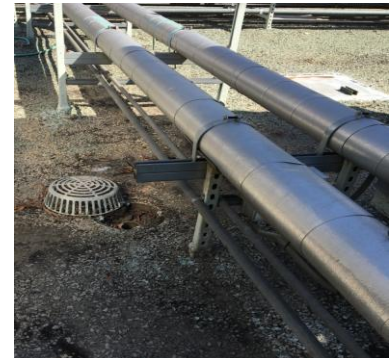
Roof drains are in poor condition.
