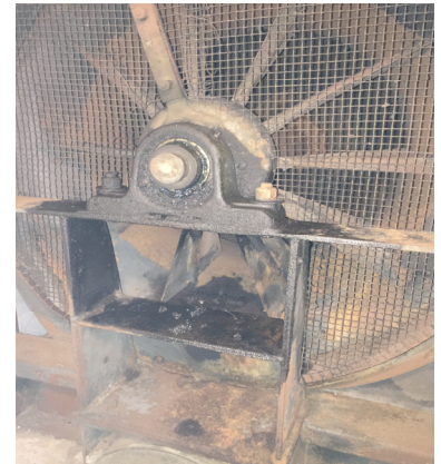
Fan station exhibits significant corrosion.
