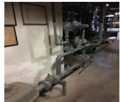
Gas meter assembly is in poor condition.
