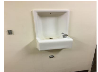
Drinking fountain is not Code compliant
