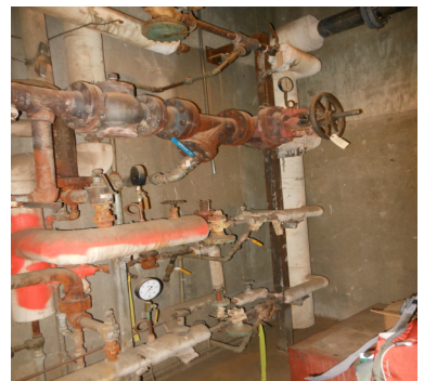
Condensate meter exhibits major corrosion.
