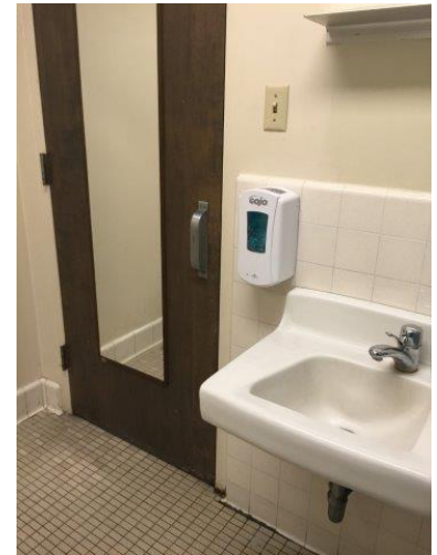
Typical Non-Compliant Restroom Entrance and Accessories
