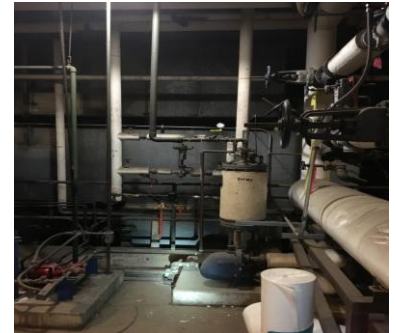
Domestic hot water generator is in poor condition.
