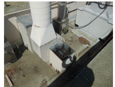
Roof-mounted building exhaust fan is in poor condition
