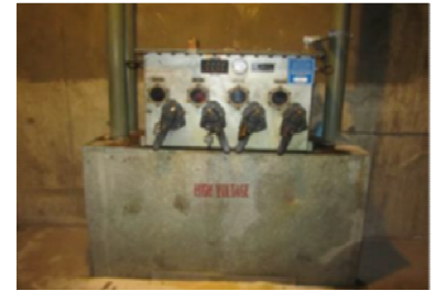
5KV Oil Immersed Switch Unit with Traces of Oil Leakage
