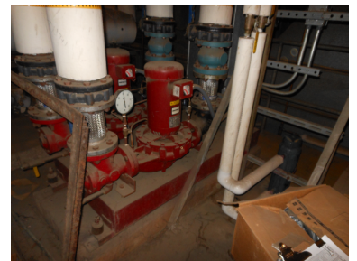
Heating hot water pumps generally are in poor condition
