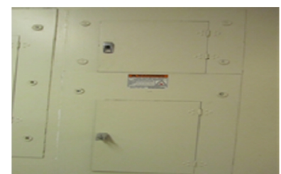
Panelboard With Broken Locks
