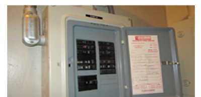
Interior of Load Center with plug-in circuit breakers & sheet metal latch
