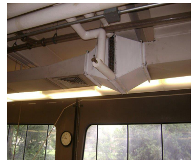
Terminal reheat coils are in fair condition
