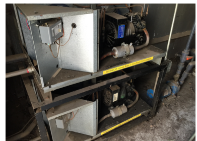
Condensing units serving cold rooms are in poor condition.
