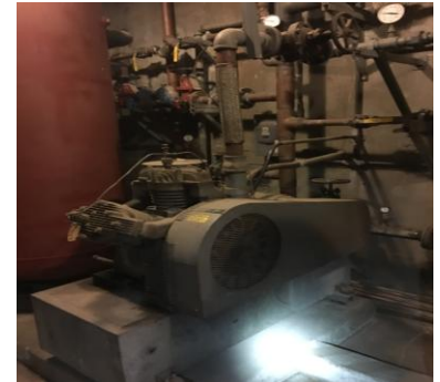
Air compressors are in poor condition.
