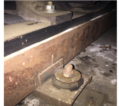
Fan station's vibration mounts and structural base exhibits significant corrosion.
