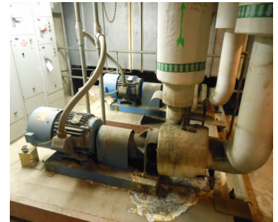
Chilled water pumps exhibit significant leakage of chilled water
