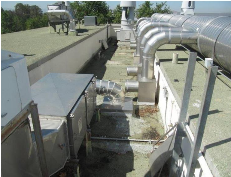
Roof Mechanical Well
