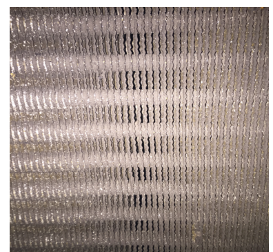
Cooling and heating coils is in poor condition.
