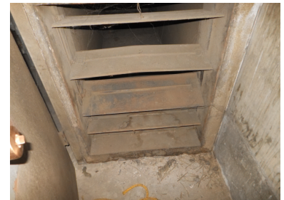
Exhaust fan damper serving the tunnel exhibits significant corrosion
