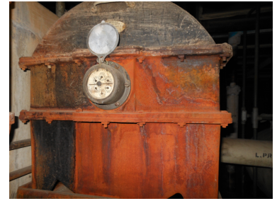
PRV station are in poor condition and exhibit major corrosion
