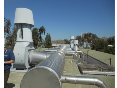
Roof-mounted fume hood exhaust fan and stainless steel manifold are in fair condition
