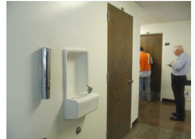
Typical Non-Compliant Drinking Fountain
