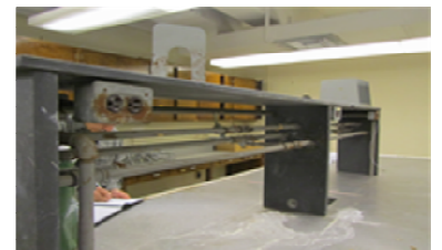
Rusted outlet at Lab bench
