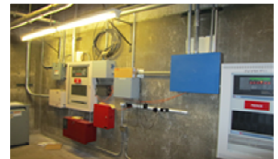
FACPs in Basement Unit Substation #1 - Electrical Room
